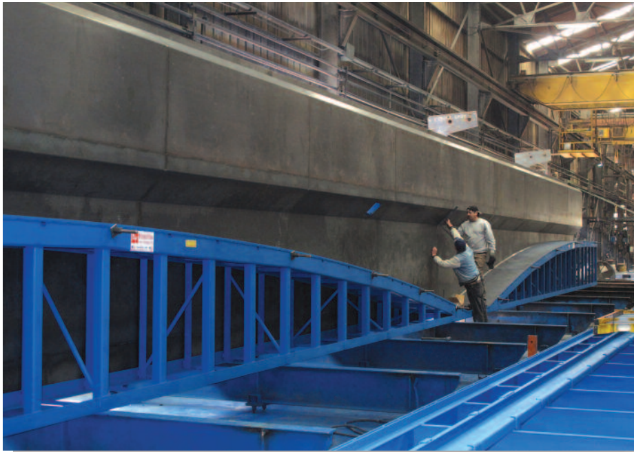
The haunch girder formwork includes an arched soffit and 10-foot, 4-inch sideforms.
