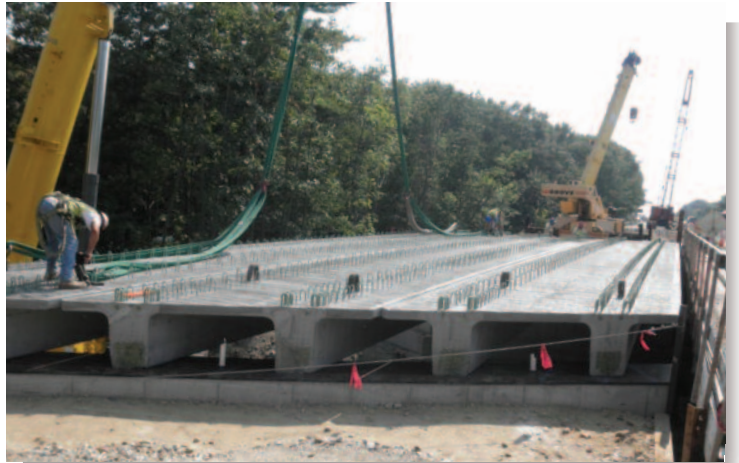
Beams act as formwork for the deck pour and provide a work platform.
