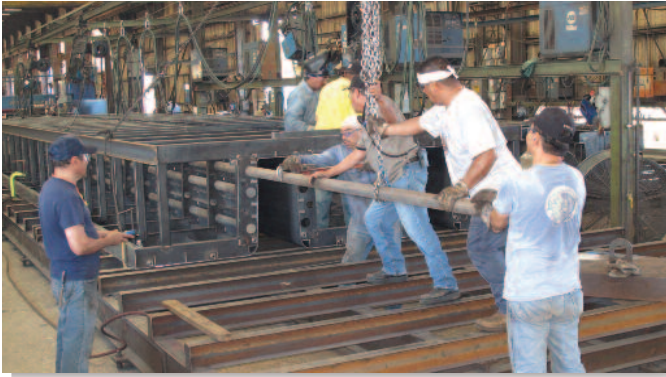
Solid steel compression bars were used in the self-stressing NEXT Beam form.
